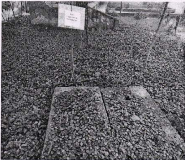
Water harvesting system
